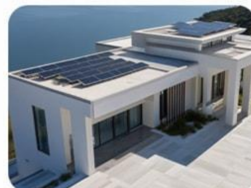
4: 光伏发电 Photovoltaic power generation
